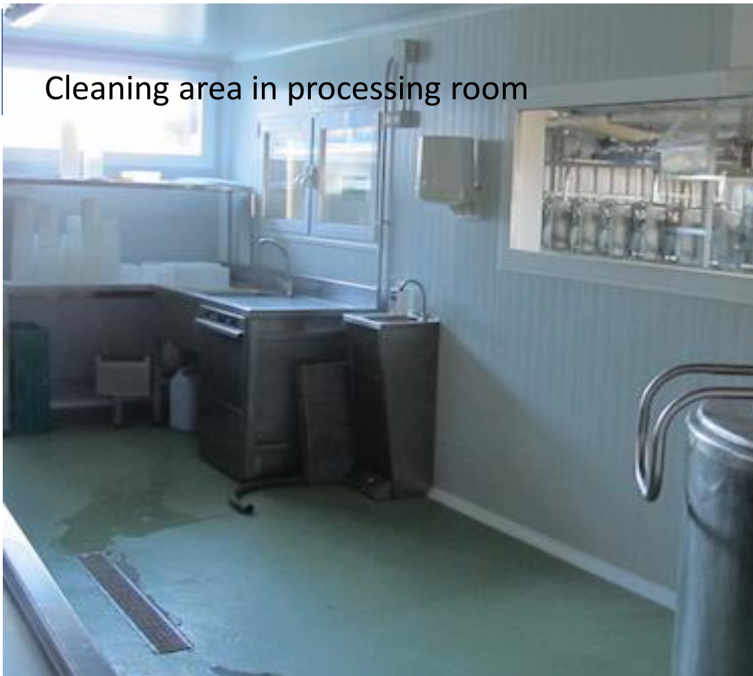
Multipurpose washbasin in processing room
